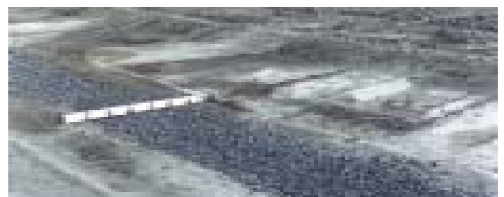
7. One of the finished underground drainage sections backfilled with 40mm clean gravel.
